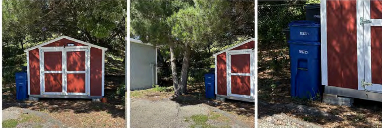
Photos(from left): View of new shed, proximity to annex and tree with overhanging branches; and combustibles, debris and open base under the structure.
