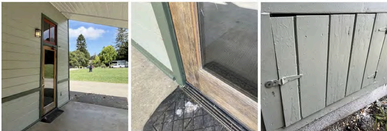
Photos (from left): Two views showing combustible wood at the base of doors and siding; and a wooden access door with a poor fit and ember entry gaps.
