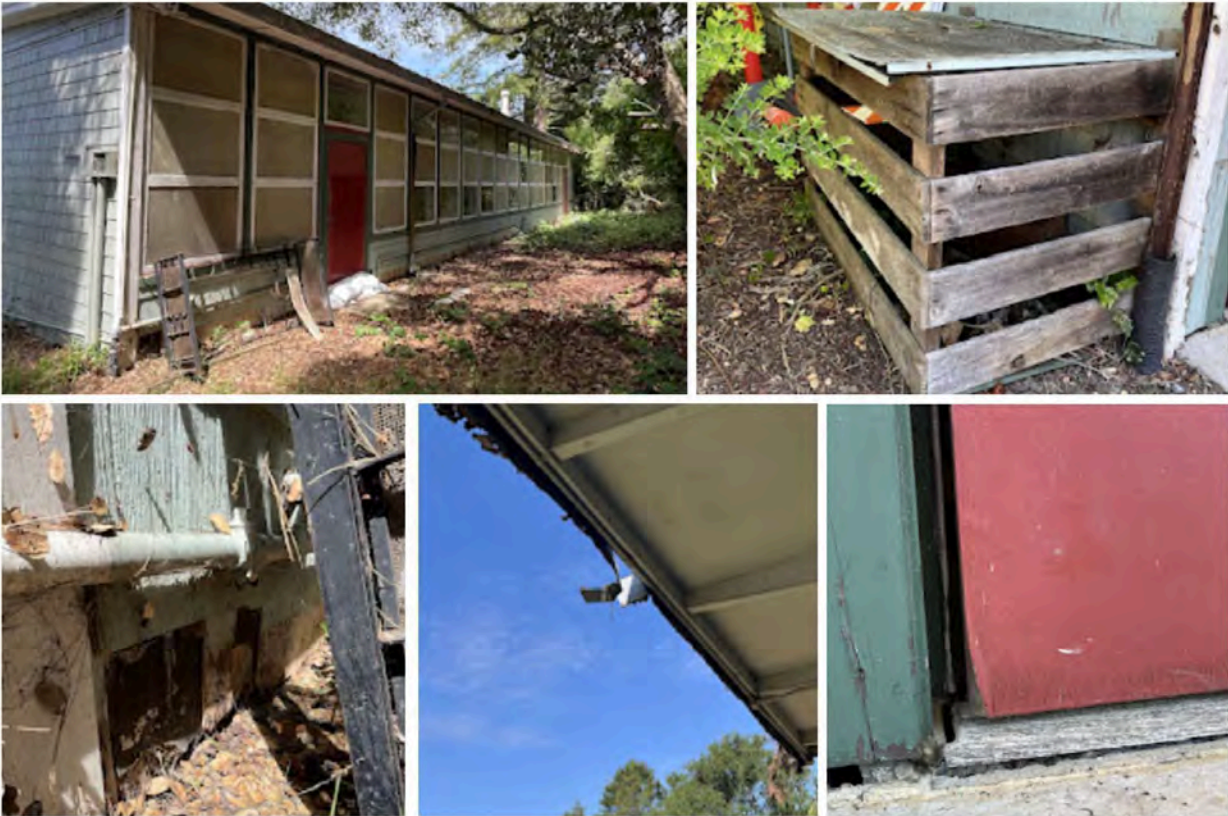
Photos: View of building from rear showing worn siding, missing windows, and multiple areas of decay.
