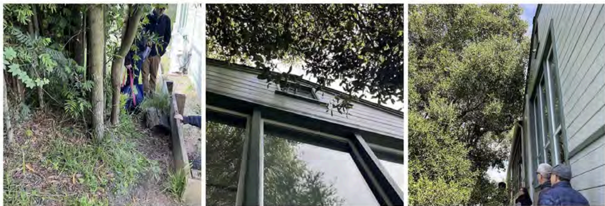
Photos (from left): cluster of trees crowding the building at southeast corner; two views of the large oak trees on west side touching the roof and gable vent, and shedding leaves and branches.
