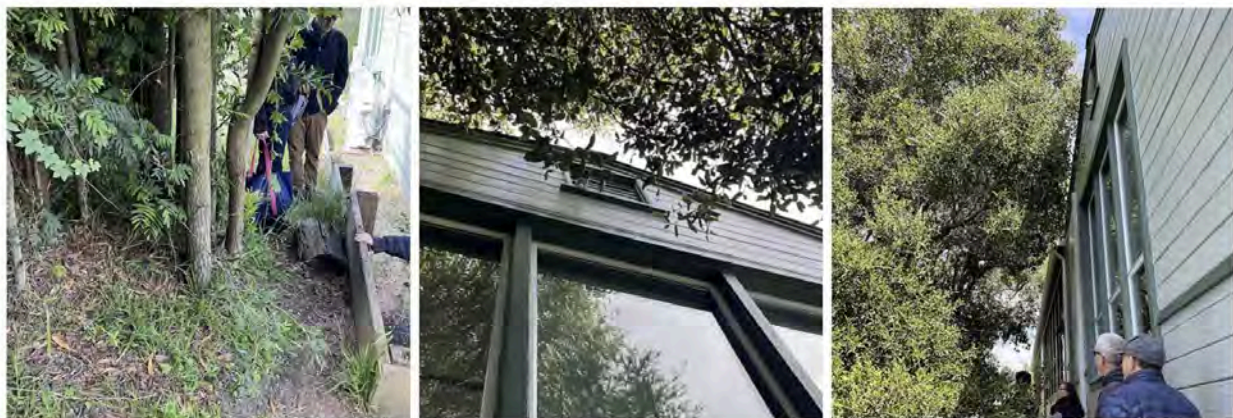
Photos (from left): cluster of trees crowding the building at southeast corner; two views of the large oak trees on west side touching the roof and gable vent, and shedding leaves and branches.
