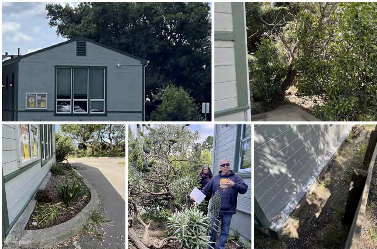
Photos (clockwise from upper left): view of trees and vegetation overhanging structure; vegetation in Zone 0 on NW corner; planter under north-side windows; overgrown vegetation on NW corner; wooden retaining wall in southeast corner prone to collecting debris.
