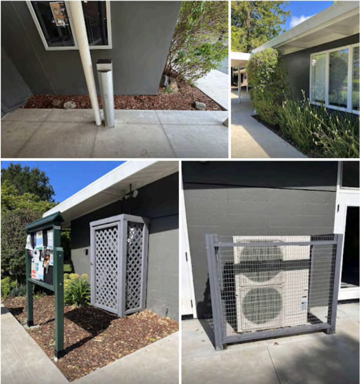
Photos (clockwise from upper left): L-shaped planter with mulch and vegetation beneath eaves at front; wooden screens for mechanical equipment on side.
